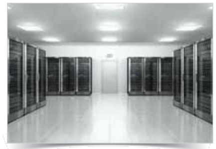
Fig.: Constant processes and highly sensitive applications such as data centres, are based on RCM monitoring.
