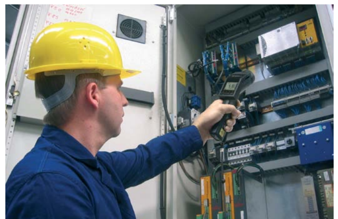
Detailed infrared temperature measurement of an electric control with the help of the installed close focus optics for 1 mm ranges of the optris LS LT
