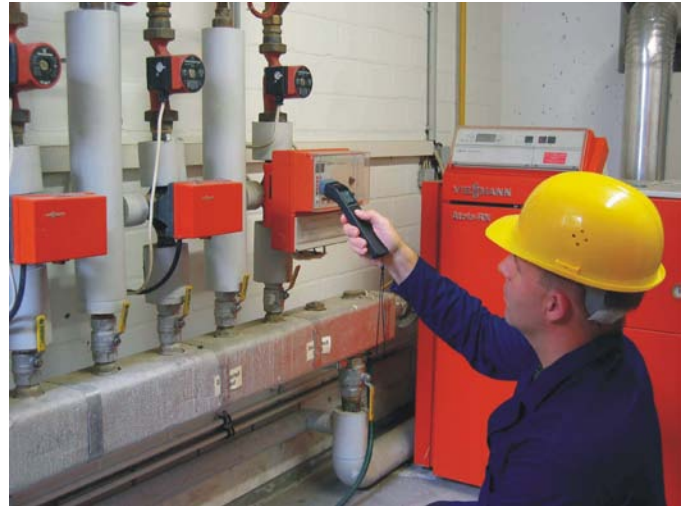
Checking the temperature of heating circles
